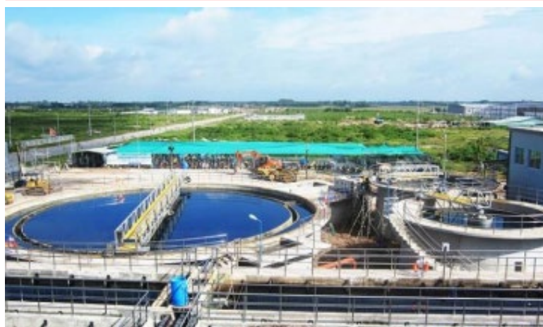
Figure 4: Water factory In Phuoc Dong IP
