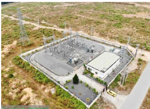
Figure 3 : Substation in Phuoc Dong IP
